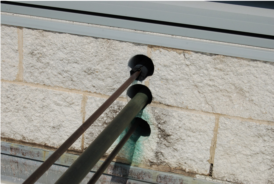
Piping penetrations through penthouse cavity-wall that was never caulked when originally constructed.
