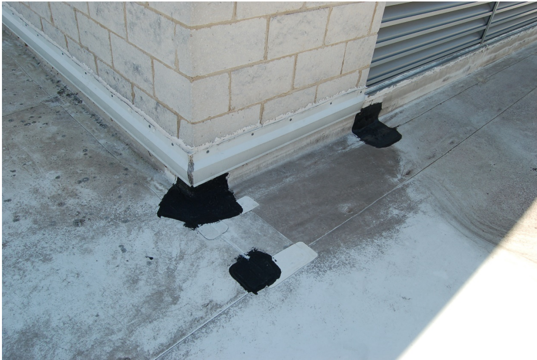
Numerous patches on classroom wing roof around penthouse where ongoing leaks have occurred.
