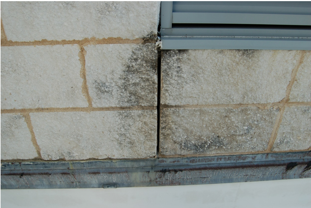
One of the cavity-wall control joints that was never caulked when building was originally constructed.
