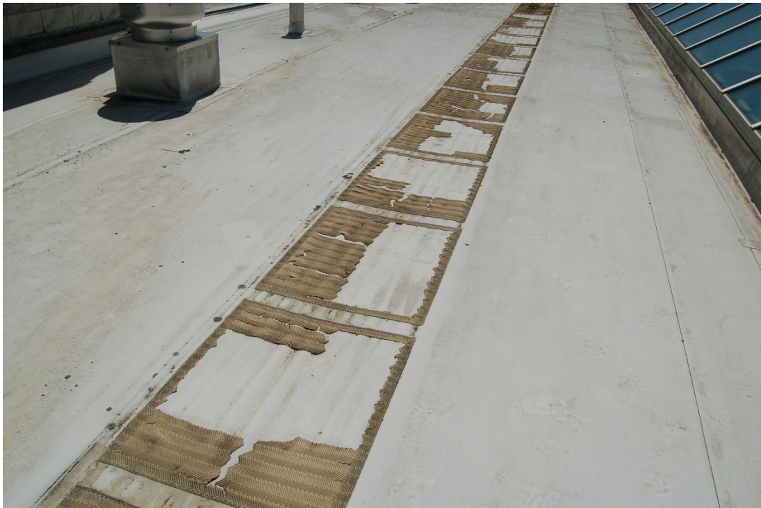
Roof walkway pads over main corridor showing signs of age.
