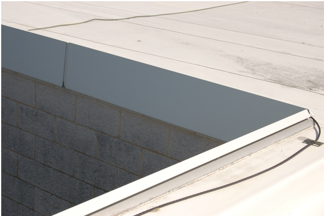
White aluminum fascia flashing installed over roofing that must be removed to replace membrane.
