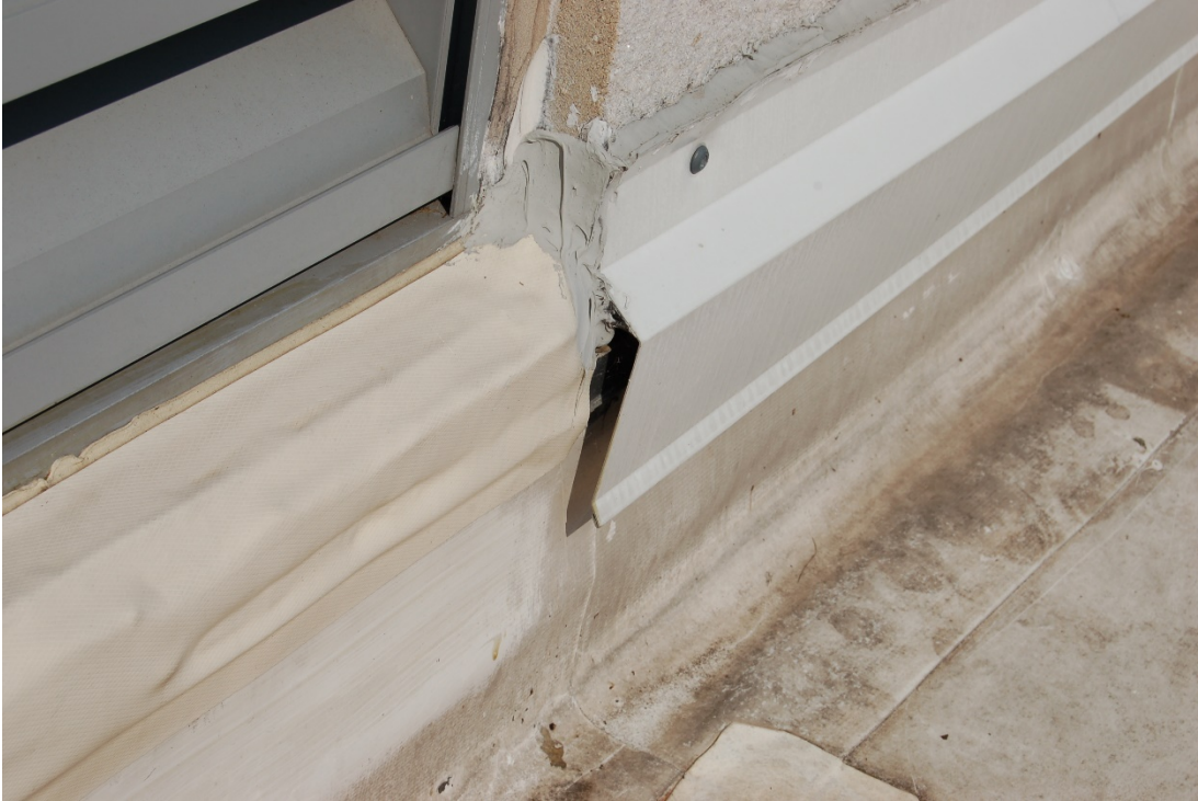
Surface-mounted aluminum flashing installed directly over cavity-wall weeps should be removed.
