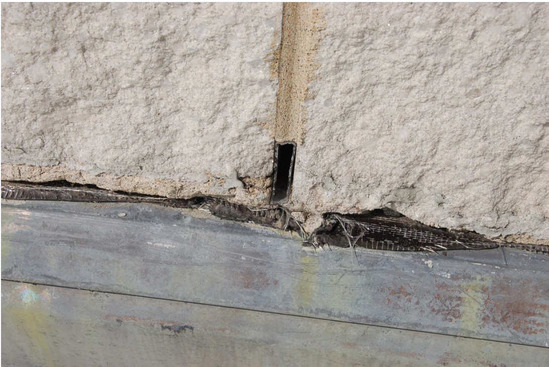
One of the cavity-wall weep holes at base of a penthouse that should remain uncovered for drainage.
