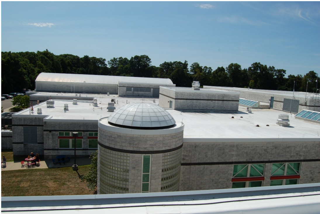
Overall view towards south showing Gym barrel-vault, gray masonry accent bands on exterior walls, and one of the three aluminum domes that must be removed to replace underlying membrane.
