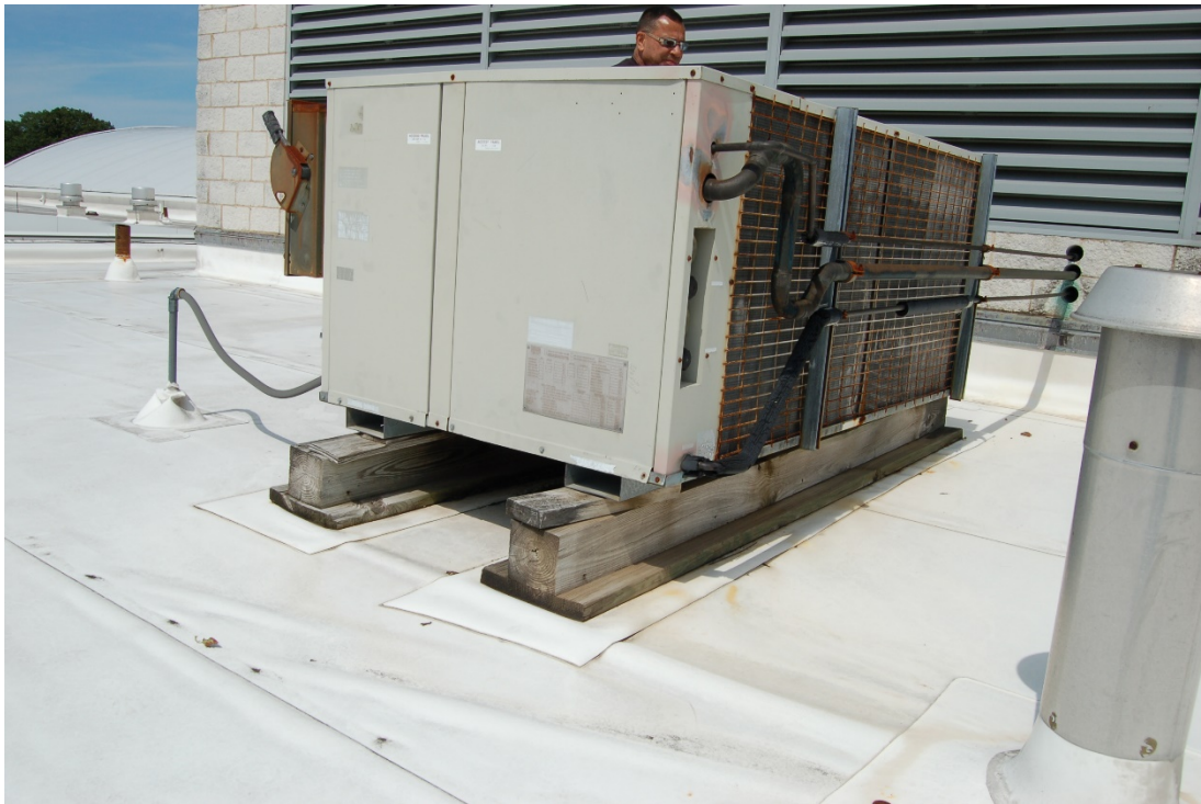
Air conditioning condenser installed on timbers loose-laid directly on membrane and insulation.
