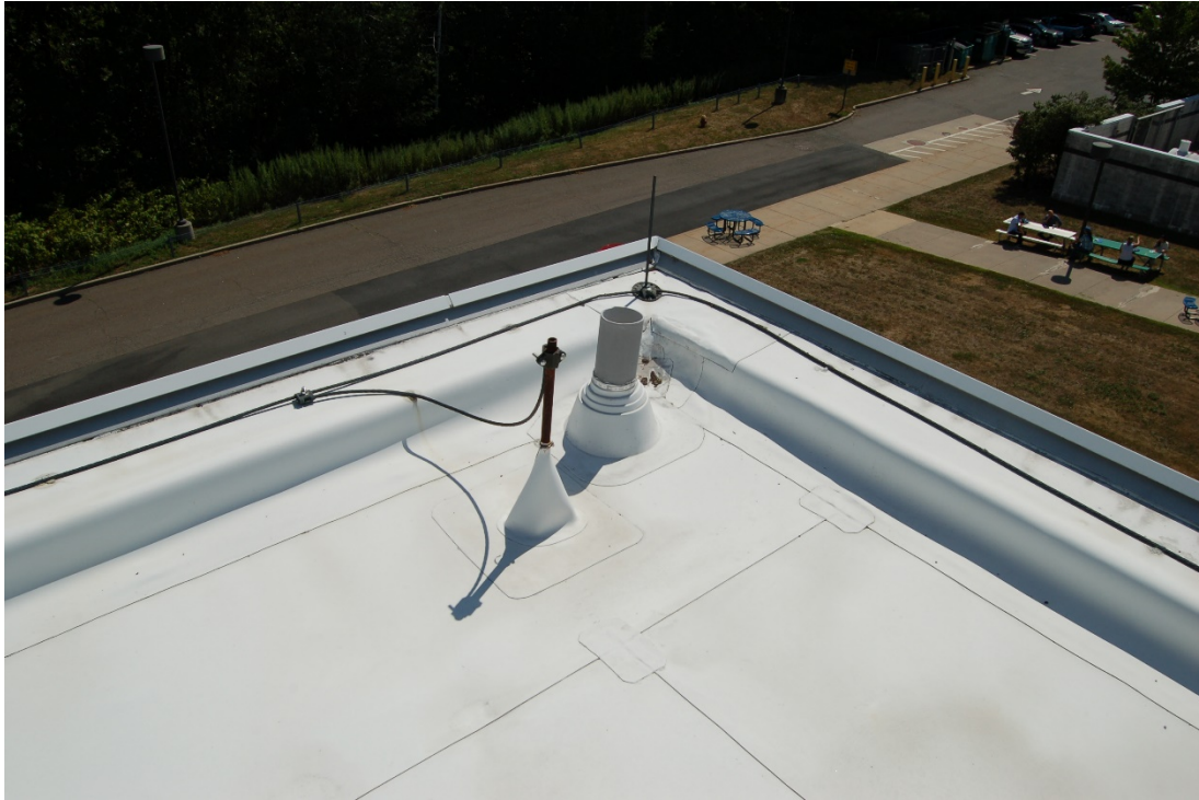
Lightning protection system installed on top of roofing that must be removed to replace membrane.
