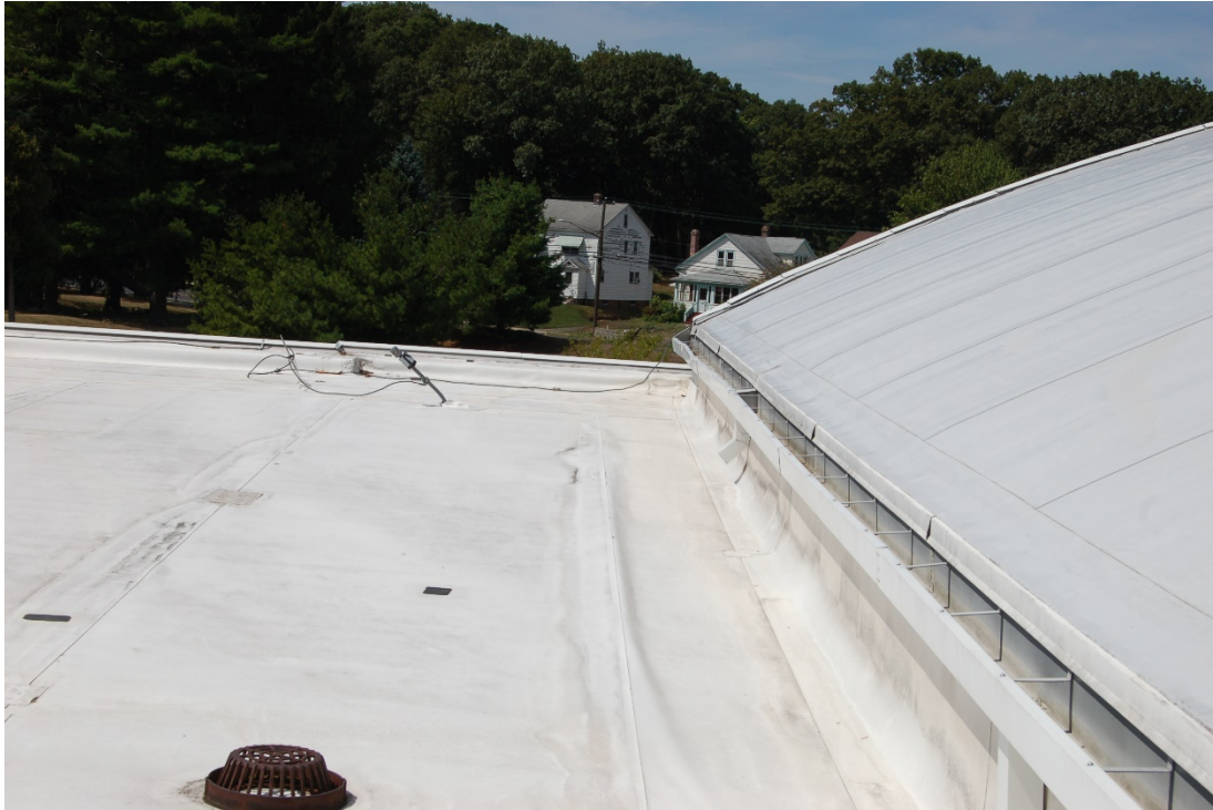
Pushed over electrical sensor conduit and torn open end of gutter showing signs of snow-slide damage.
